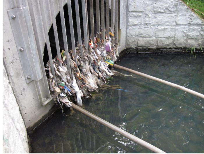
Stormwater outfall from C St. to Chester Creek (Northon, 2012)
