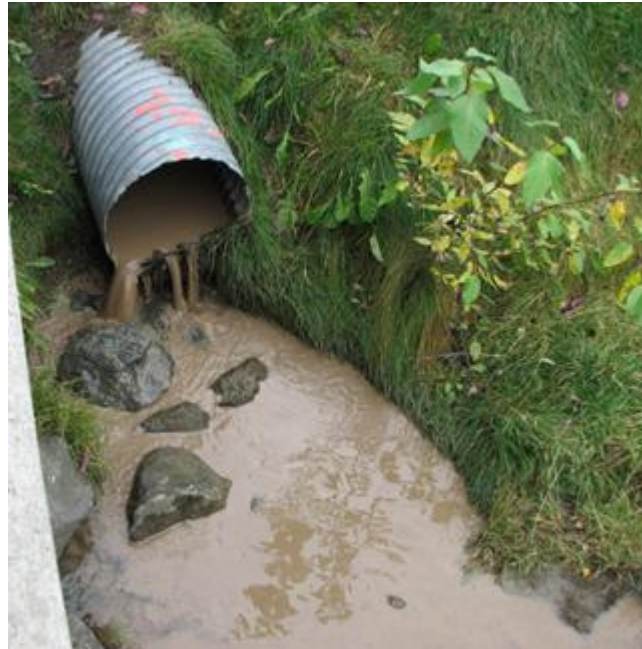
Stormwater outfall with high sediment load from a construction project at 52nd and Lake Otis flowing into Campbell Creek (Northon, 2007)
